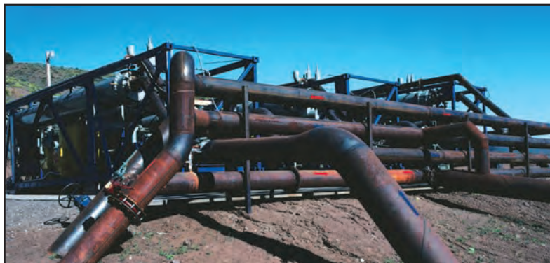
FIGURE 1. Large, capital-intensive projects throughout the CPI typically require complex piping arrays. Thoughtful planning is required to maximize efficiency and minimize risk during the acquisition, supply, fabrication and erection stages required for such piping arrays, especially in the face of changes elsewhere in the project design
